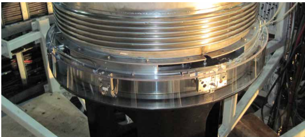
Mounting configuration of the ERA 8400 angle encoders on the telescope drive system for azimuth positioning
